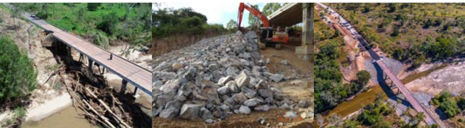
Image (l-r): Damage to Alice River Bridge N&FN Monsoon Trough, reconstruction process, ariel view completed works.
